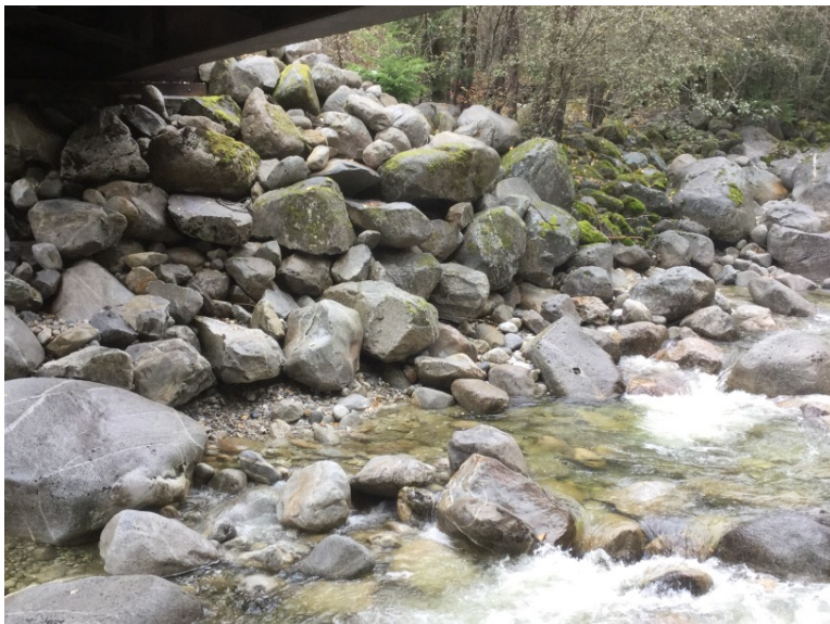
Upstream right bank riprap appears oversteepened
