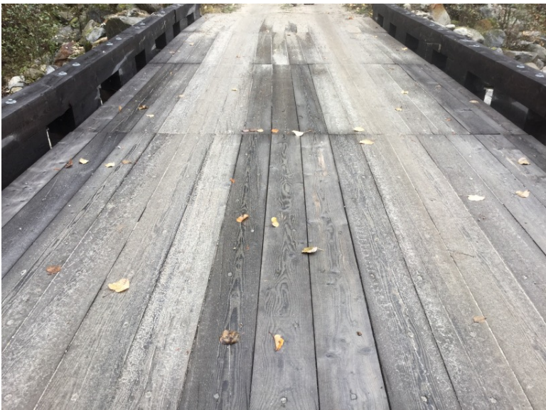
Deck panels slightly misaligned
