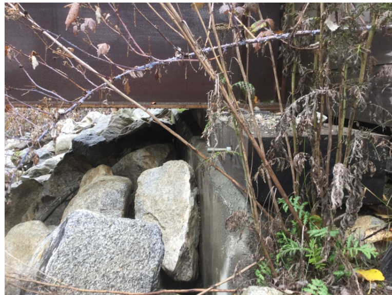
Timber sill at left bank is skewed to lockblocks
